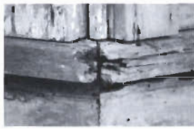
This rotted - and irreplaceable - woodwork...
