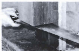
10" rotted bottoms of these load-bearing columns...
