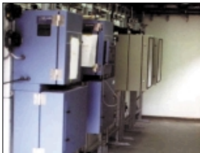
■ Figure 4. Example of a standardized analyzer house.
