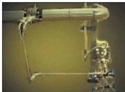
■ Figure 1. This installation causes errors and increased maintenance.
