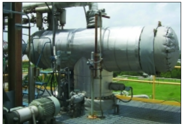
Typical overhead condenser installed on a vacuum distillation column.
