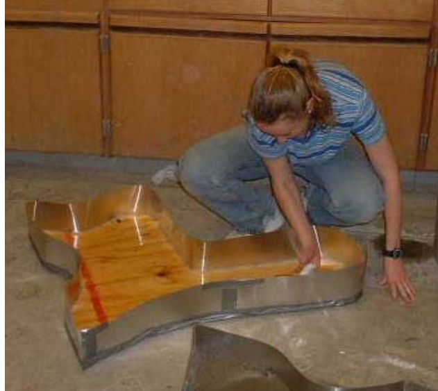
NYWEA Member Lindsey Wilkins finishes off the molds for the concrete ends of the benches.
